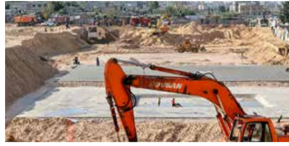
Egyptian diggers and earth movers work at the construction site of a new housing complex north of Gaza City.
